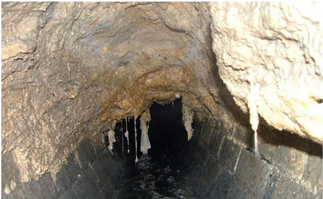
FIGURE 2: FOG CLOGGING A SANITARY SEWER
