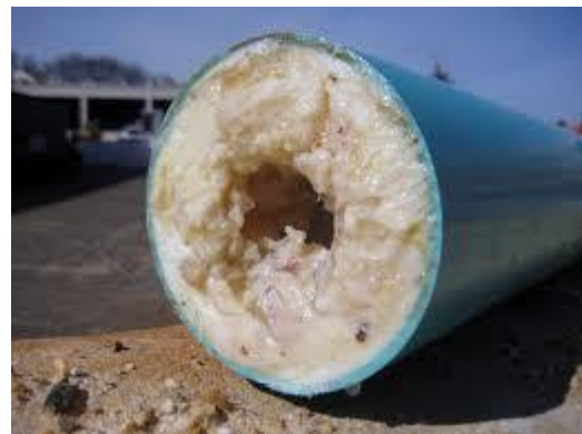
FIGURE 1: FOG CLOGGING IN A PIPE
