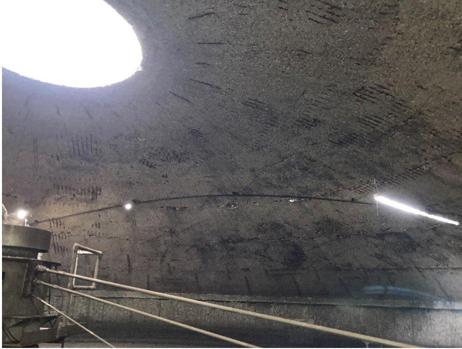
Welded mesh rebar has lost concrete cover. Two holes in the concrete cover can be seen with light coming through between the two light fixtures.
