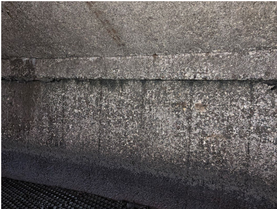
Trickling filter walls have experienced surface deterioration but are in better condition than the dome.
