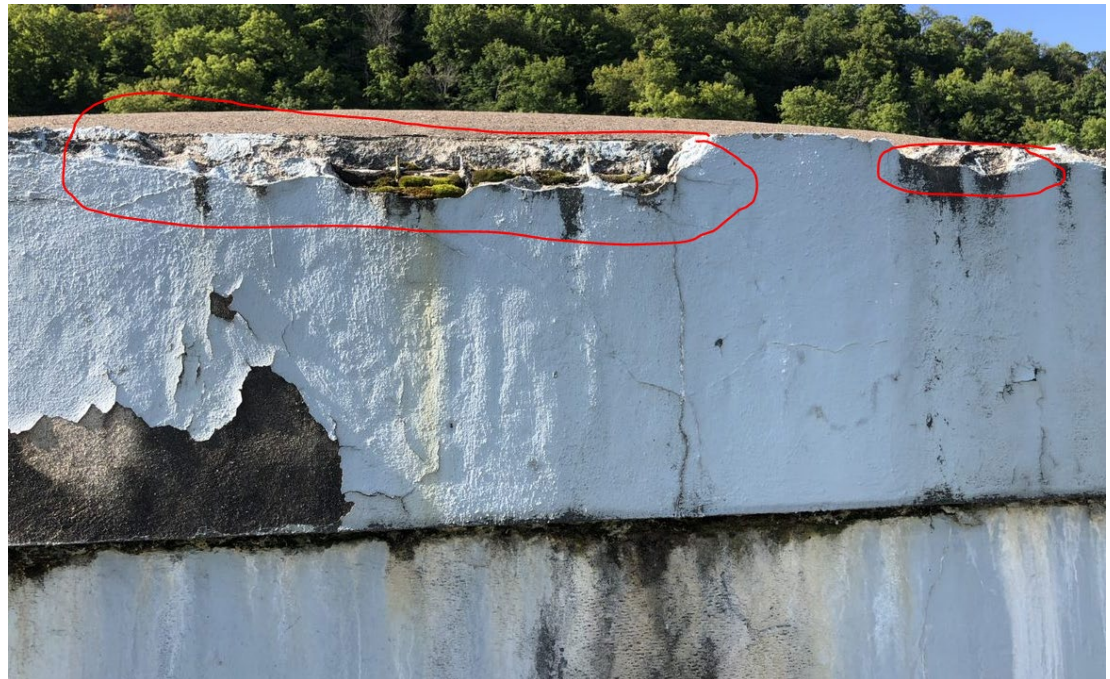
Figure 5 – Trickling Filter Exterior
