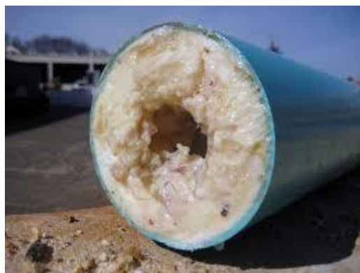
FIGURE 1: FOG CLOGGING IN A PIPE
