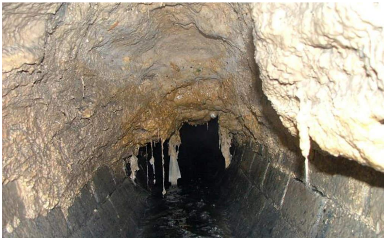
FIGURE 2: FOG CLOGGING A SANITARY SEWER
