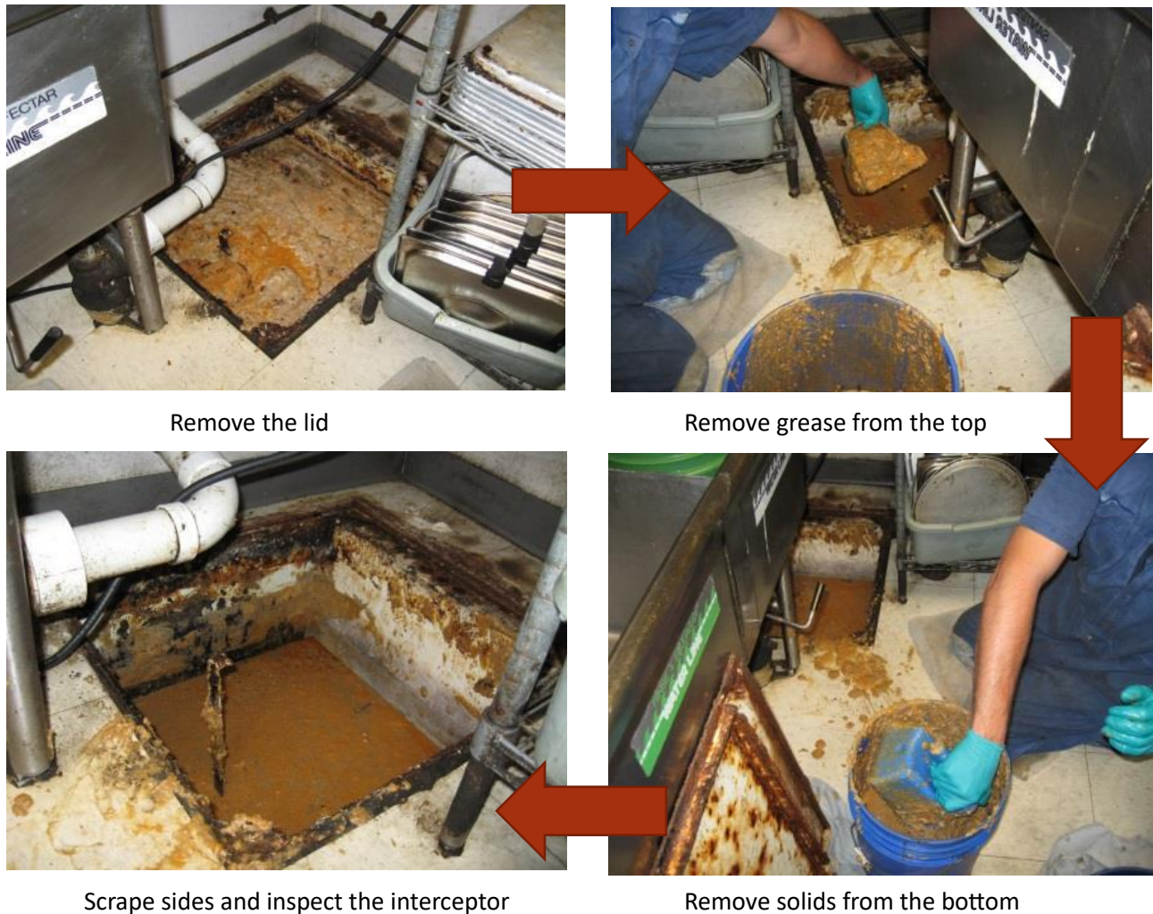
FIGURE 5 CLEANING A HYDROMECHANICAL GREASE INTERCEPTOR
